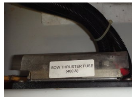
Above, an example of labeling fuses with their function and their amp rating. Below, a selection of spare fuses.
