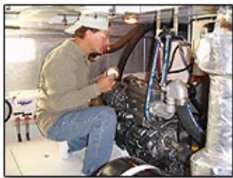
John performs an engine room check
